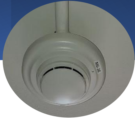
Typical Suite Smoke Detector
