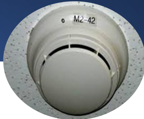
Typical Building Fire Alarm Smoke Detector
